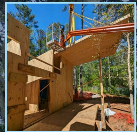
The KPNC's new environmental education building will showcase cross-laminated timber or CLT.
